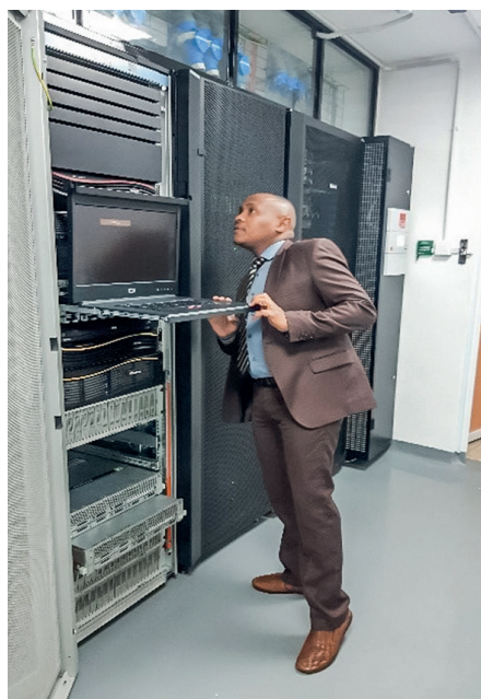
The Manager, ICT, Mr. Alex Kangethe at the newly installed server room equipment in Kawi Complex
