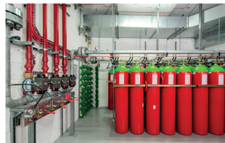
Data Centre Fire Suppression Systems
